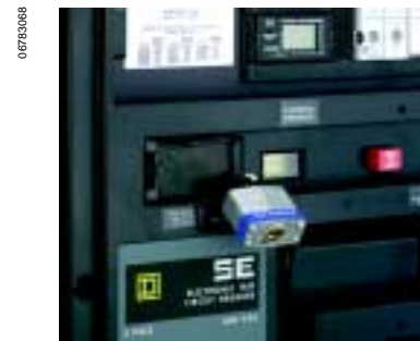
Padlocked Drawout Mechanism
